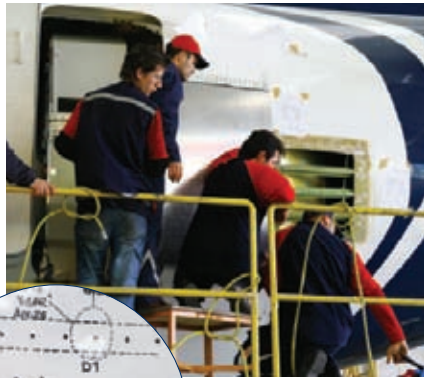
This 737 arrived at myTECHNIC with a large number of dents around the rear door caused by ground support equipment. As this was outside Boeing's repair limits, the Turkish company developed its own repair scheme that was approved by the OEM (photo: Ian Harbison)
